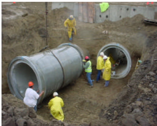
Westside Inter-tie (above and below)
