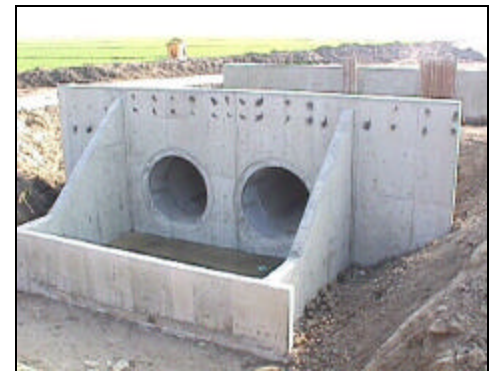
Two 72" Outlets from Lateral #4 into Inter-tie Canal
